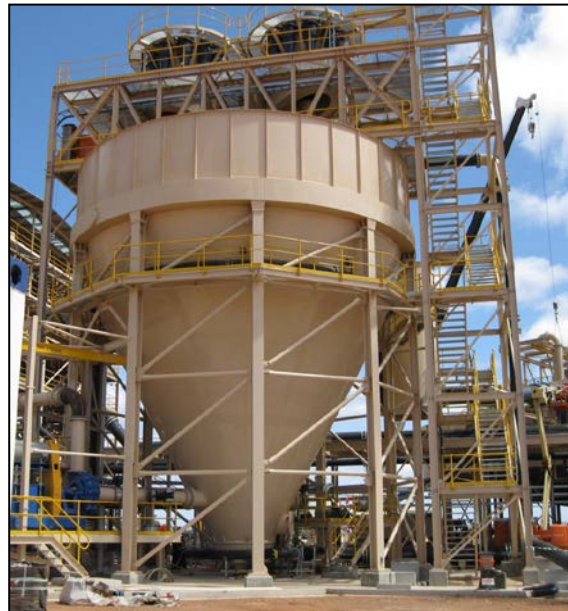
Figure 1: Surge bin in service
